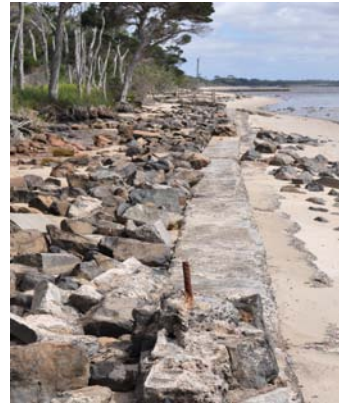
Malcolm Drive seawall ruins
